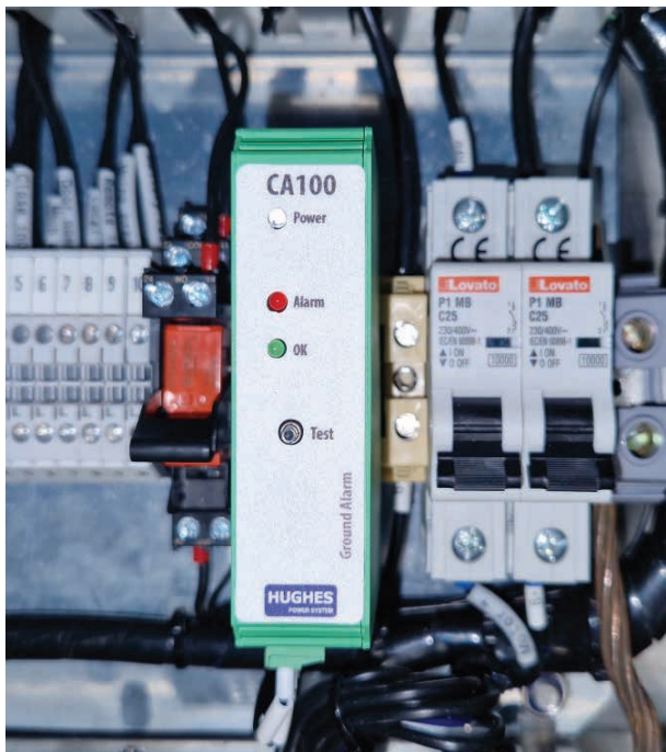
Installation in the motor drive cabinet
